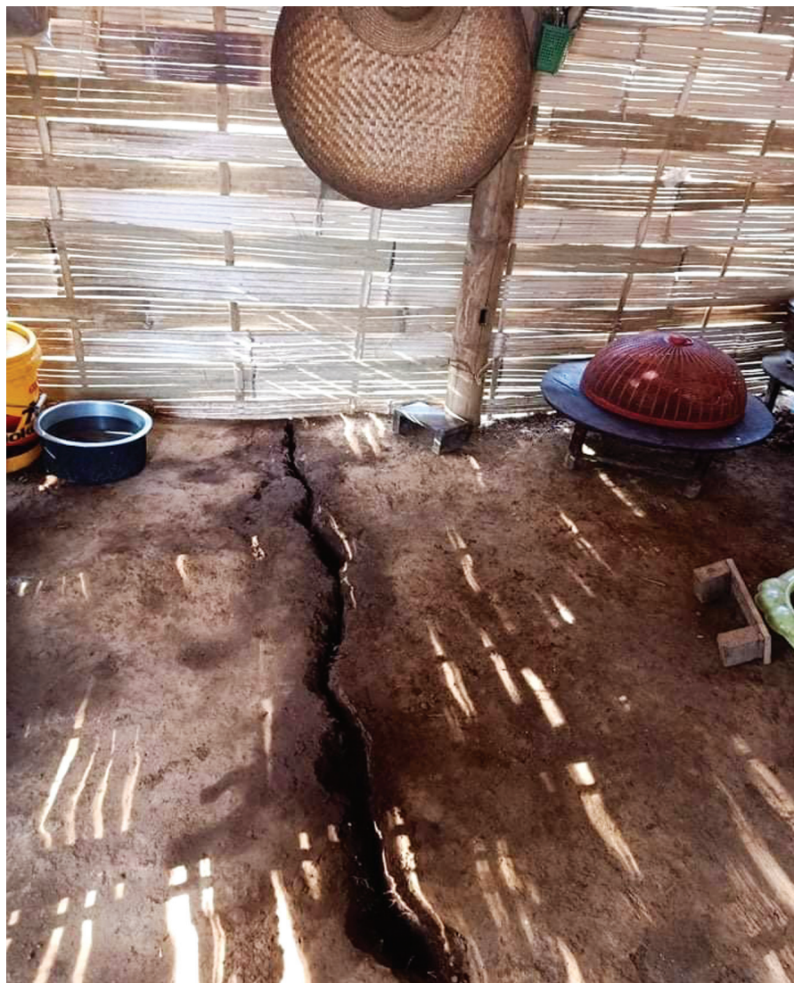
^ Landcracks in villager's house in Tak Liet
