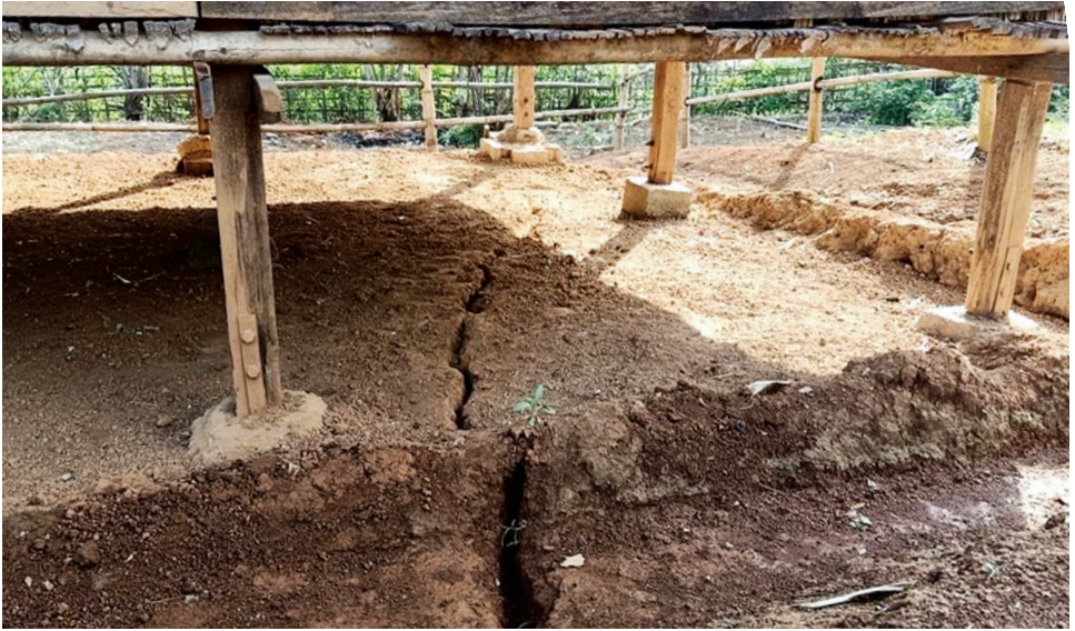
⤴ Land cracks under Tak Liet villager's house
